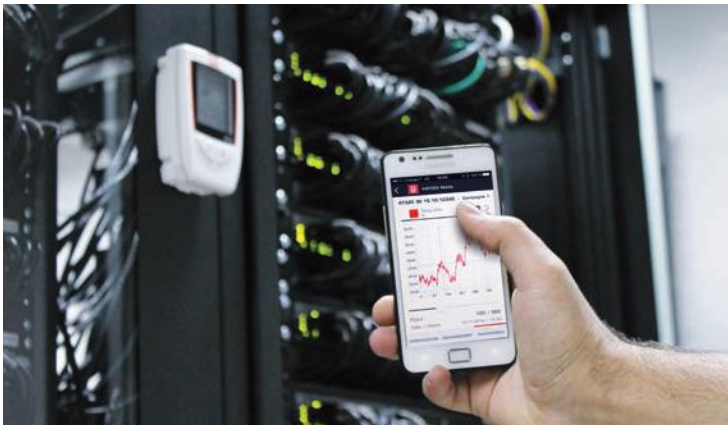
Control of climatic data from a data centre using the smartphone application
